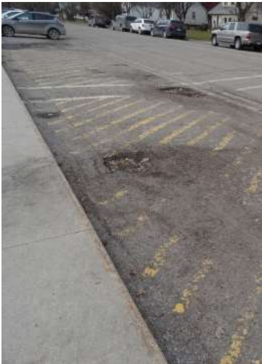
Area in front of Magelssen Elementary in the summer showing a maintenance need.
