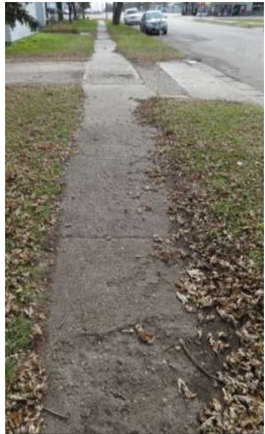
A local sidewalk showing a need for maintenance and repair.
