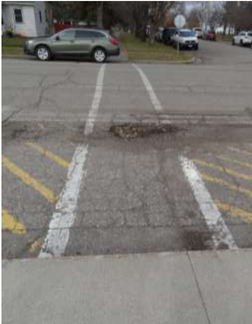
Crosswalk near the school showing a need for road repair and crosswalk alteration.
