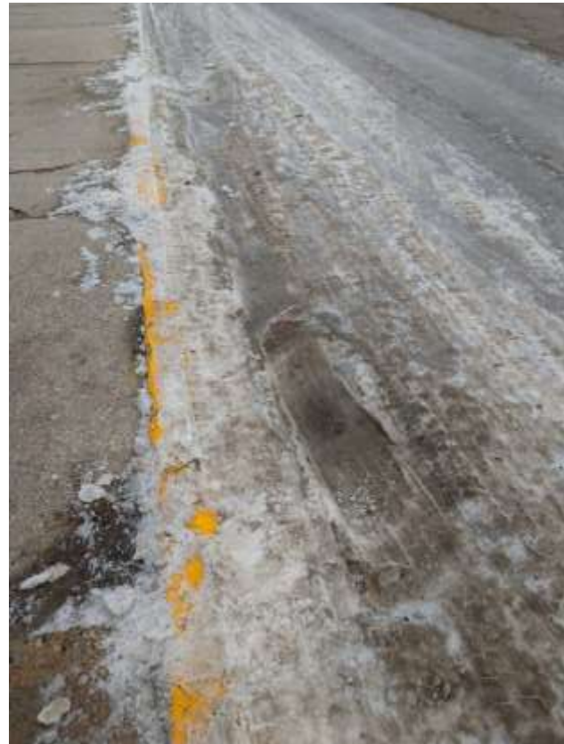
Area in front of Magelssen Elementary in the winter showing drainage, ice build-up and other winter issues that cause maintenance issues in the summer.
